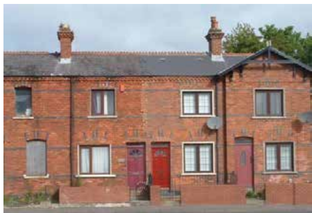
Shore Road, Whiteabbey Extended window opening, inappropriate size and configuration with redundant soldier course lintels over openings
