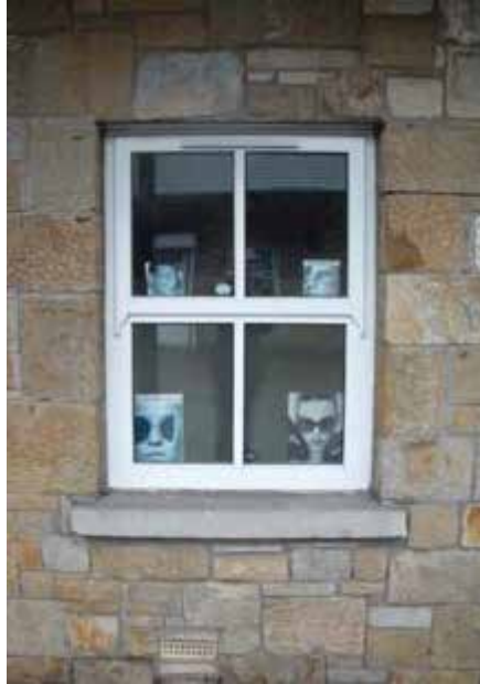
Buttermarket, Fivemiletown Sliding sash windows replaced with top hung casement windows (replete with ‘ornate’ horns to upper casement sash!)
