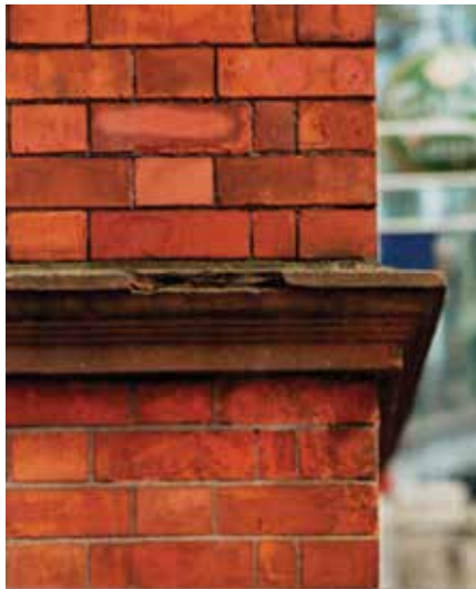
Late 19th- / early 20th-century smooth red brickwork: note the regression in the pointing above the stone string course and the modern cement pointing below
