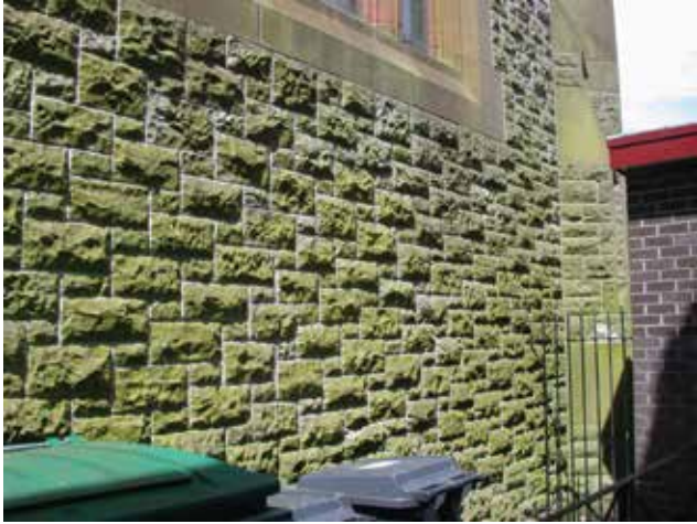
Extensive 'greening' of sandstone (Photo courtesy of C. Adamson)
